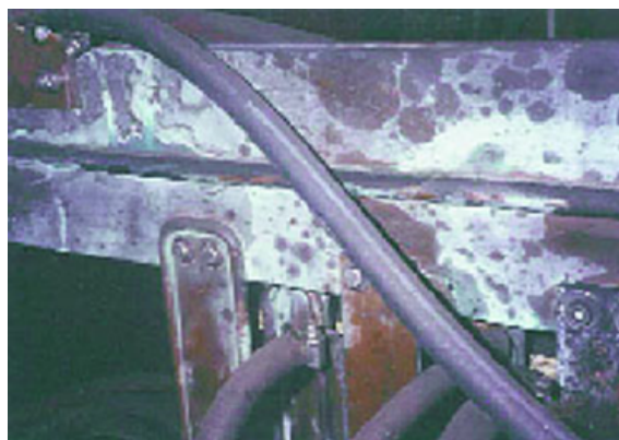
Collector bus shows signs of heating and possible condensation; bus section at lower right shows signs of overheating
